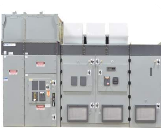
MV Motor Control and Drives
